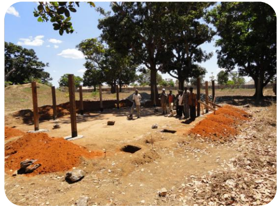
A small pavilion we are building to host the many meetings and seminars we have around Montepuez.
