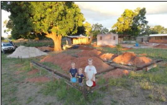
Luke, Andrew and Joshua pause to pose in front of the future site of our teacher house where the foundation has been poured.
